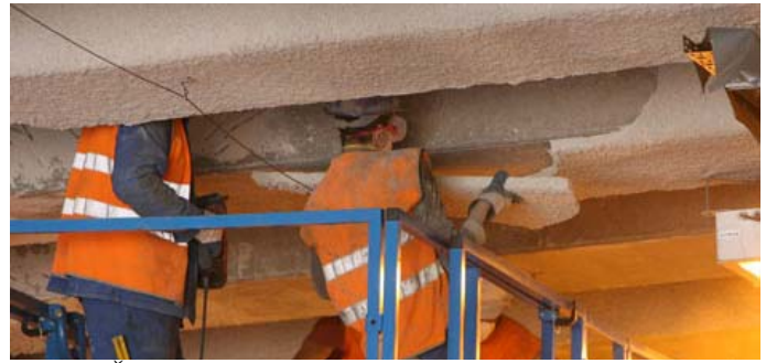
Gallery Šentvid; removal of vermiculite fire protection. Bonding layer on the left side remained on concrete (white latex), on the right side bonding was absent or it remained on fire protection.
