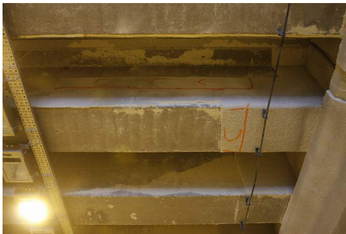
North portal of tunnel Šentvid: Beam construction of old gallery with marked area with loose vermiculite fire protection
