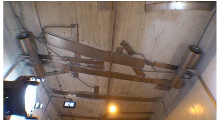
New gallery of tunnel Šentvid: water leaks; fire protection coating was installed on stainless steel drainage.
